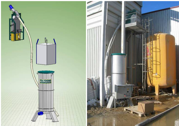
Fig. 4: Fully integrated dosing system for micro-polypropylene fibres (Line 9, Metro Barcelona)
