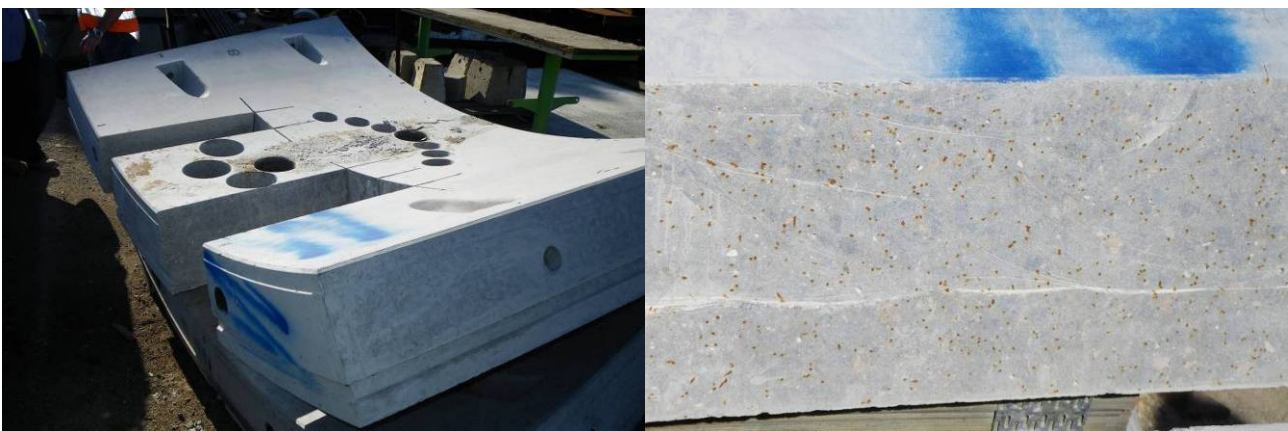
Fig. 6 Weather exposed sample segment from trial casting for outfall tunnel segments (Victorian Desalination Plant project, Melbourne)
