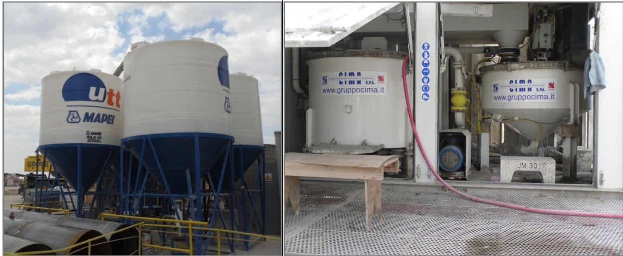
Figures 8A and 8B. The images show the storage tanks (8A) and batching plant (8B) of the back-fill grout components at Hydraulic tunnel “Arroyo Maldonado” job site.
