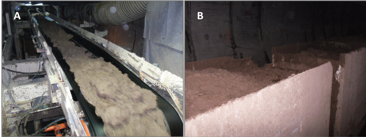
Figures 5A and 5B. The figures show the ground conditioned on the muck transportation systems at the job site. 5A Shows the conditioned ground at the transportation belt. 5B. Shows the ground conditioned once at the transportation trucks.
