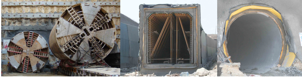
Figure 2: Tunneling works of Kirazli-Basaksehir-Olimpiyat metro line, Istanbul. From left to right; exit and transport of two TBMs in 750 m long Ikitelli Sanayi station, cut & cover tunnels near Olimpiyat station, NATM used near Ziya Gokalp station.
