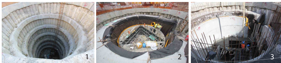
Figure 5: Important manufacturing stages of an evacuation shaft. 1- pile insertion and excavation, 2- construction of shaft lining, 3- stairwell construction.
