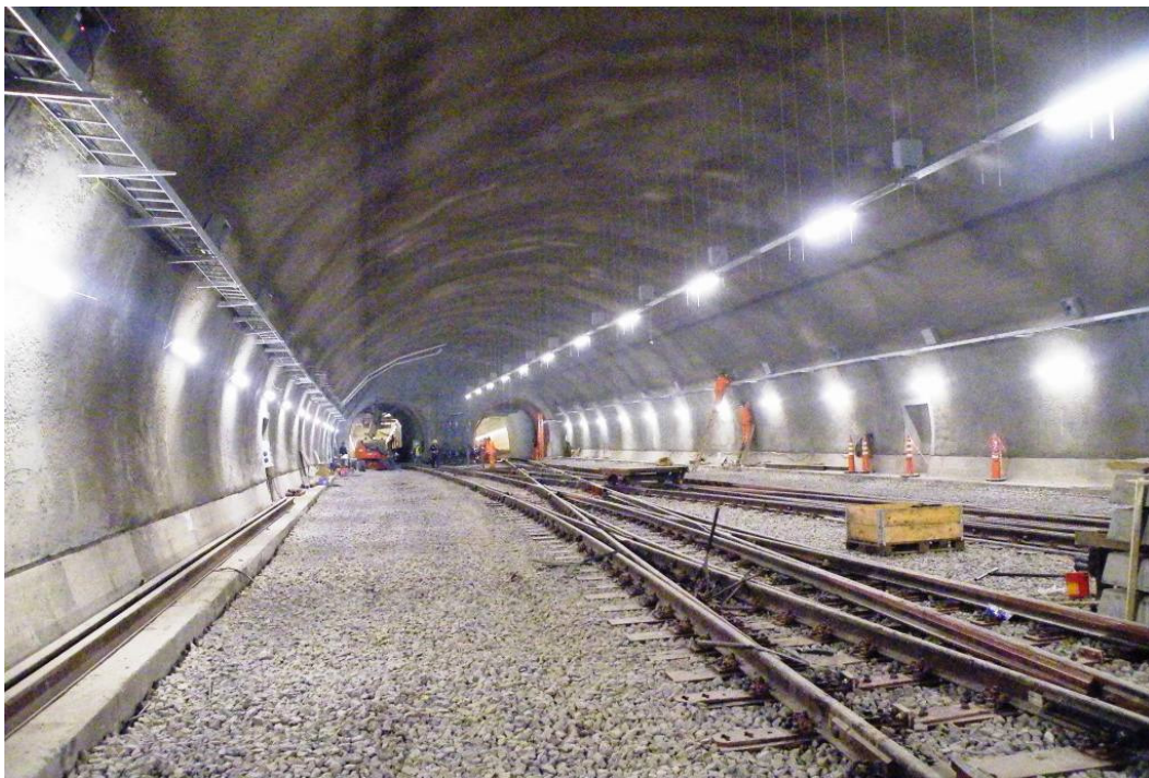
Figure 7: Buenos Aires Line B garage cavern
