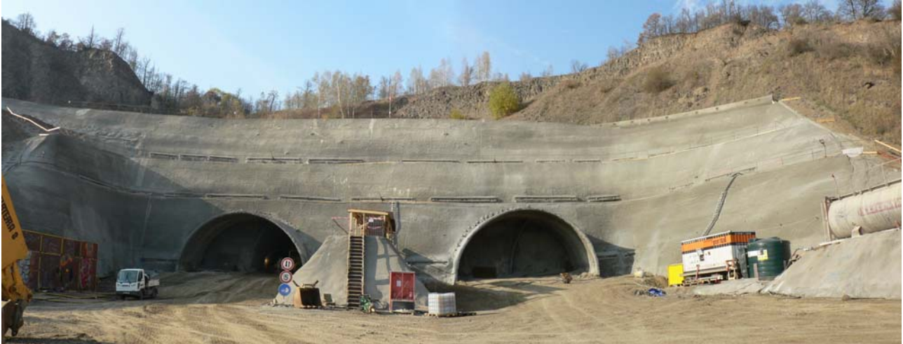
Fig. 5 View of the Prague's portal with the surcharging concrete block between tunnels
