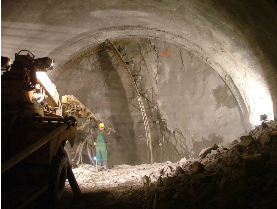
Figure 6: Required rockbolting on face and starting steel support arch in case of divided top heading in rock class IV (Váró & Kandi, 2011)
