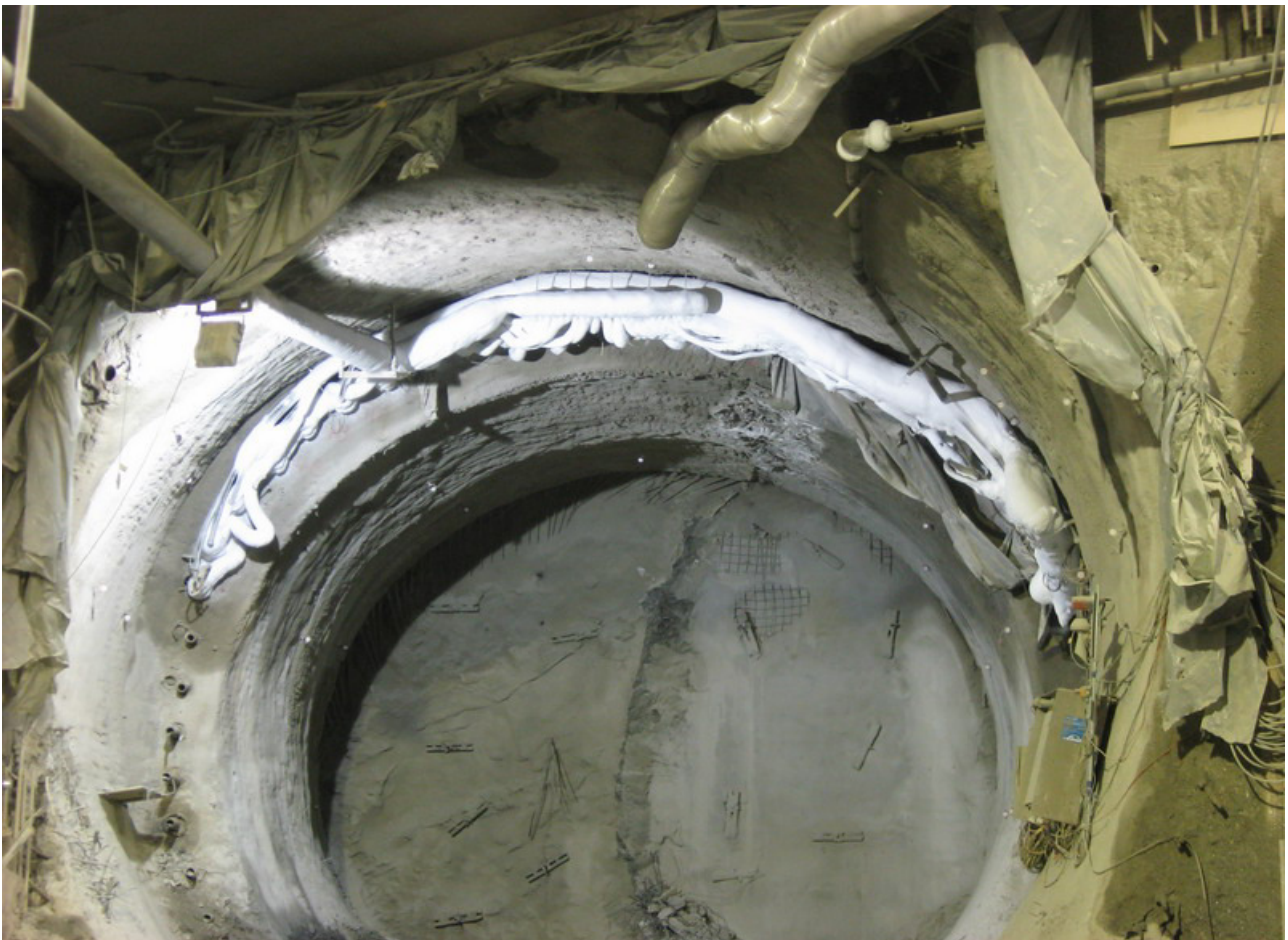
Fig.5: freezing at south platform tunnel
