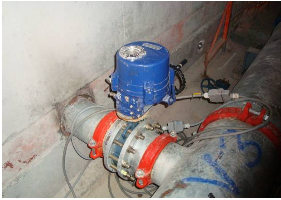
Fig. 17 Actuator on valve ballast tank (BGFL, Korea)
