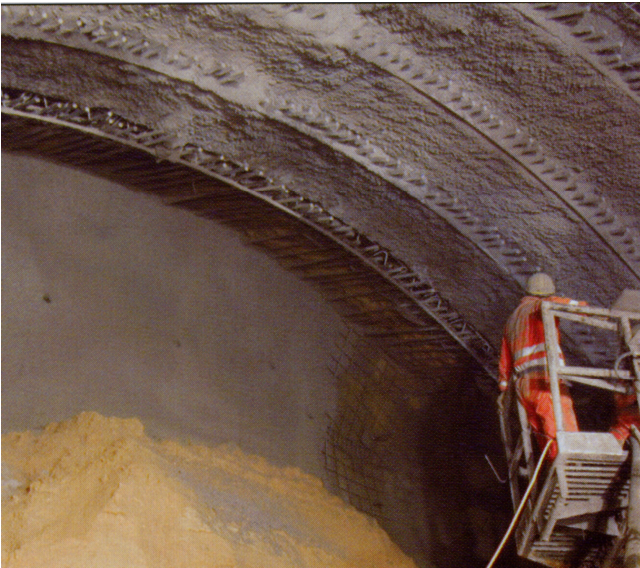
Figure 1. Spiles installed through the lattice girder to the face in every excavation step.
