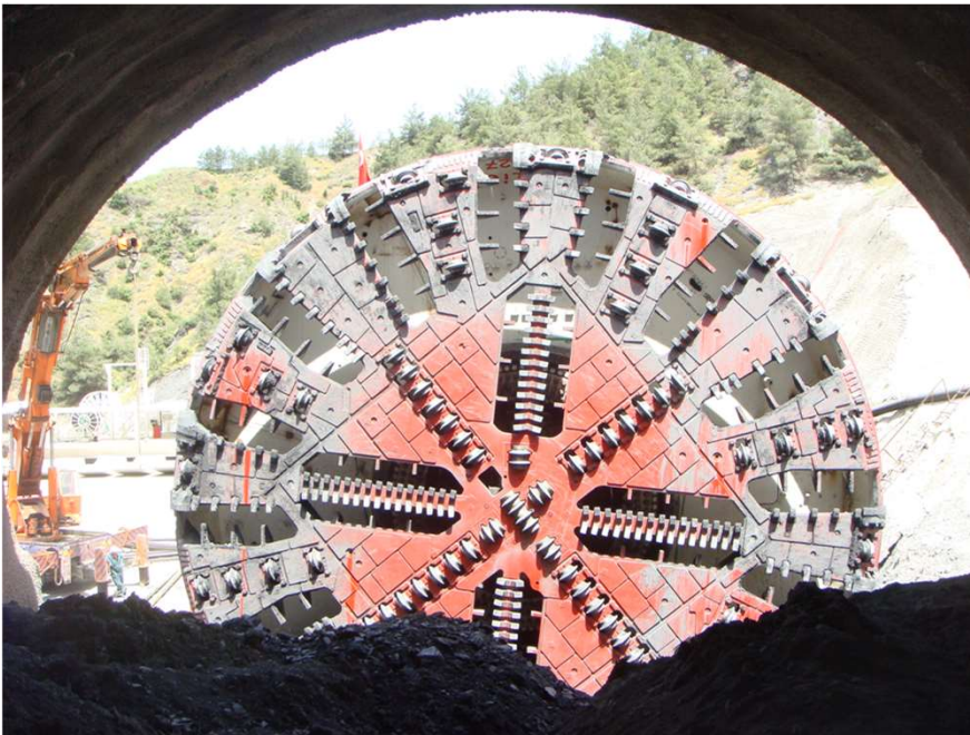
13.7 m diameter Single shield TBM
